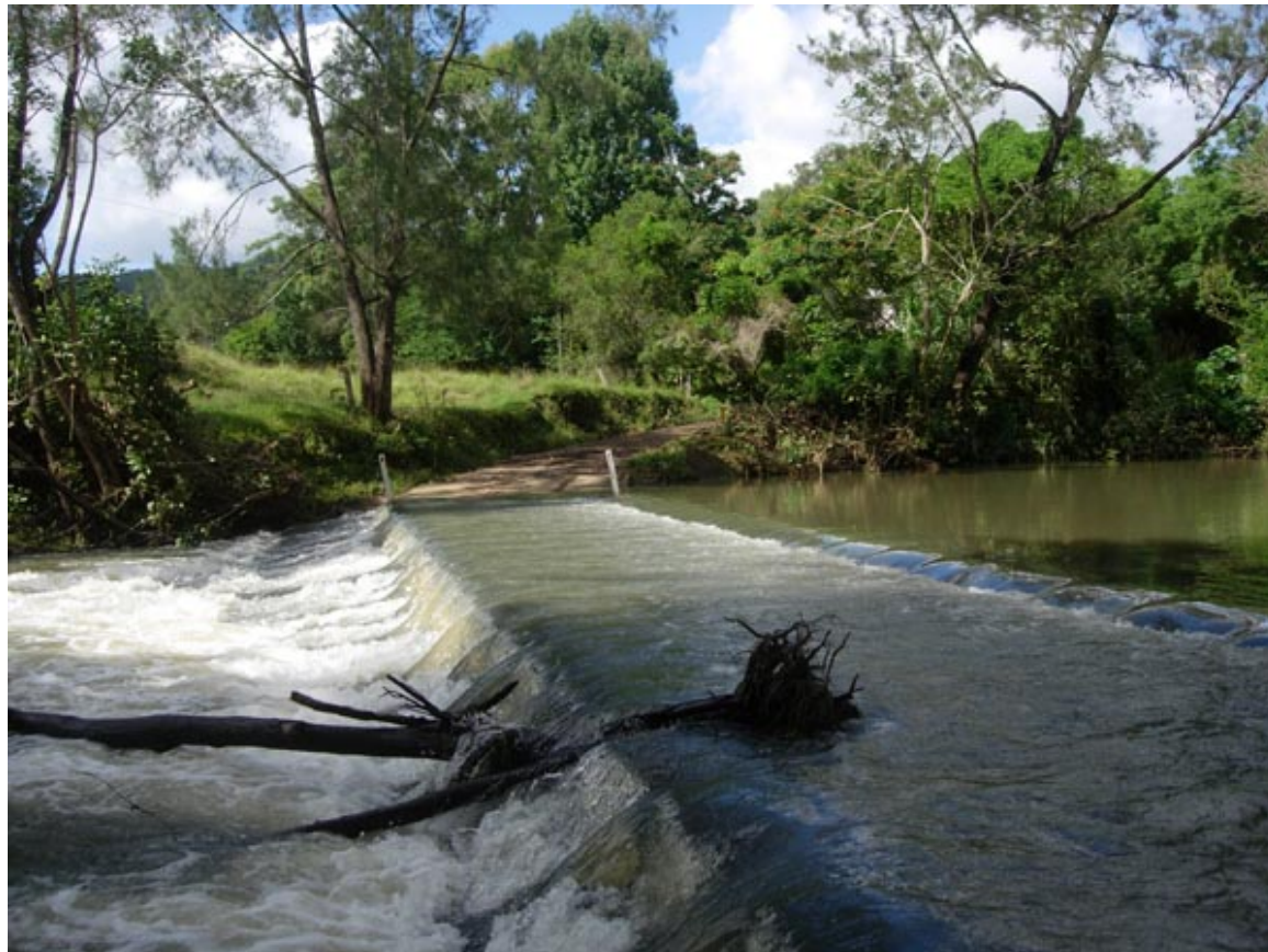
left: the causeway on Chillcott Road. Water depth on the causeway in this photograph, was about 40cm.
