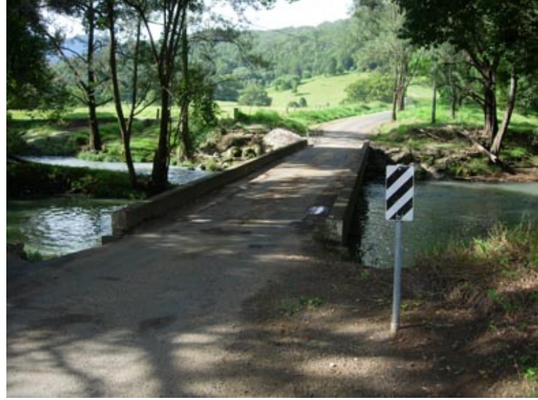
below: the Hopkins Creek Road bridge is 300 metres south of Numinbah Road, 2 kms west of Chillingham
